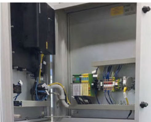
Assembly and wiring
